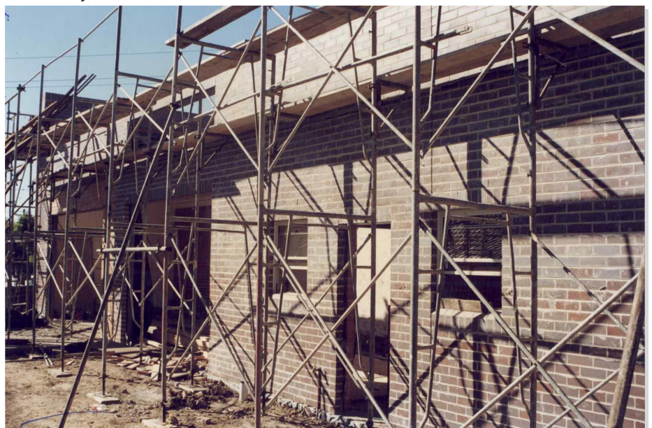
SDN Hurstville during construction, 1996. The front section was kept but the rest was rebuilt. Source: SDN Archive
